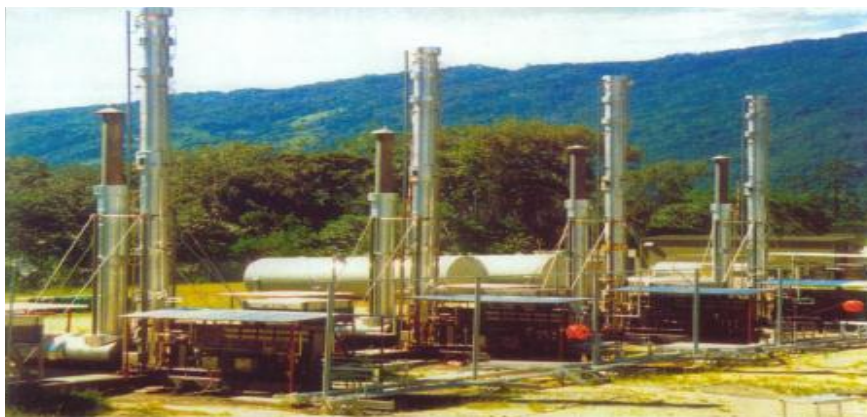
Figure 2: 150BPD Mini-refinery located at Papua New Guinea. ( www.minirefinery.com )
